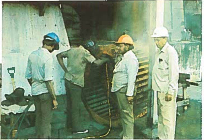
Welding repairs being effected to an induced draught fan used in our boilers.
