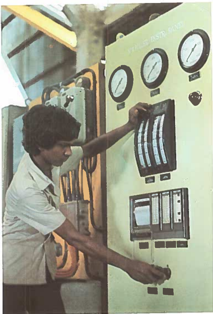
Many young men have found responsible jobs in the industry and perform efficiently, as this young man who works at the No. 1 Boiler Instrument Panel at Skeldon.
