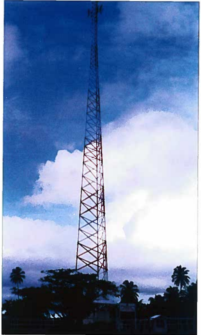
This voice and data communications tower was erected to facilitate a communications link among the Corporation's locations. Speedy access to information and data can increase the efficiency of the sugar industry.
