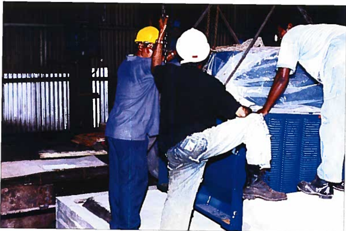
Ensuring the production of 300,000 tons of sugar annually, involves major factory rehabilitation and a reliable supply of cane: a turbo alternator set being shifted into position at Wales Estate.
