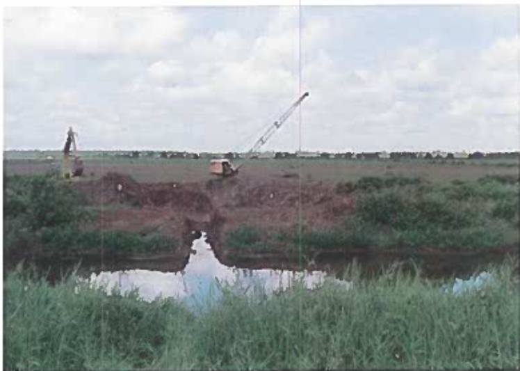
Establishing drains at Port Mourant United, part of the expansion programme on stream at Albion\Port Mourant Estate.
