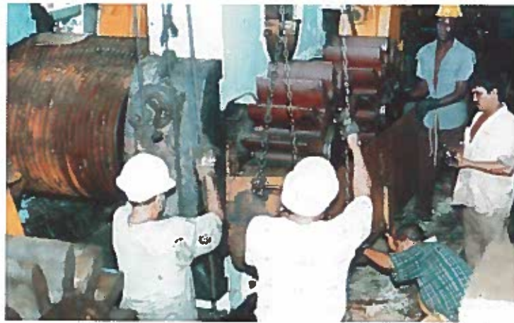
Rehabilitation of Mills is part of the Out-of-Crop maintenance programme planned for the Estates.
