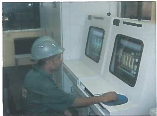
DCS System in Operation
