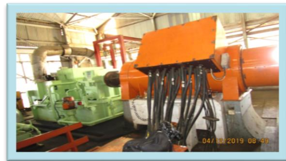
Uitvlugt Estate Power Generating Engine
