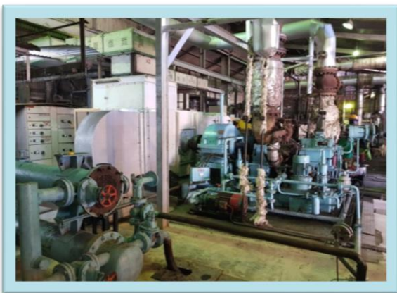
Blairmont Power Generating Engine – 2.5 MW
